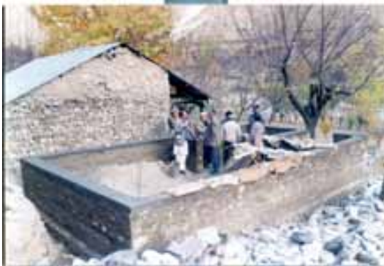
Fig.6: Improved construction techniques being implemented for earthquake resistant rural houses, after 1991, Chitral earthquake
