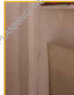
Cracks in column of interior spaces
