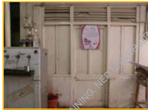
Damaged ventilator at ground floor
