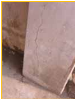
Cracks in column
