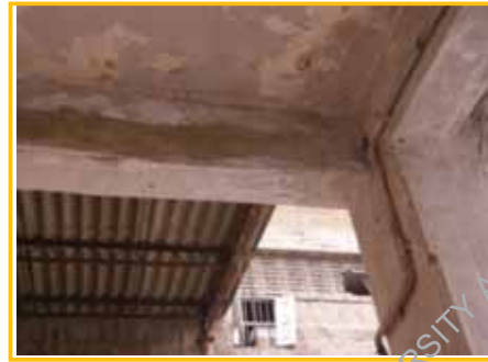
Cracks and Seepage stains on roof slab
