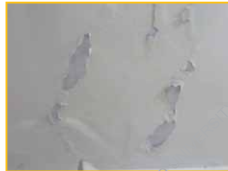
Peeled off Ceiling Paint
