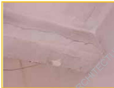
Cracks in beam
