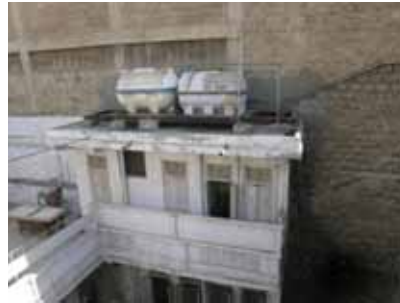
Fibre glass water tanks placed on the roof top of second floor
