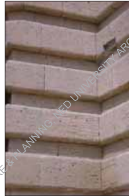
Figure 59. Damaged Stone Surface
