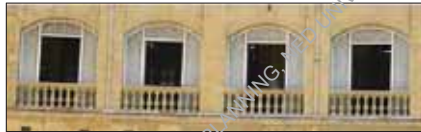
Figure 40. Added Jaffery in the Arch Openings
