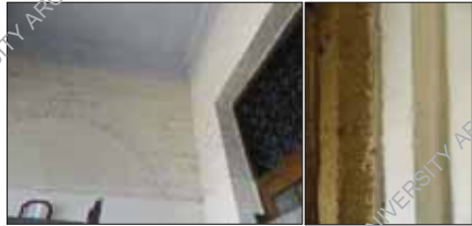
Figure 48 (a, b). Paint Coat on Stone Walls
