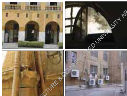
Figure 86 (a, b, c, d). Dirt Accumulation and soiling of various surfaces
