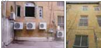
Figure 42. Exposed AC Units Figure 43. Exposed Electric Wiring
