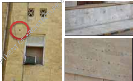
Figure 72 (a, b, c). Holes and Cavities at Various Locations
