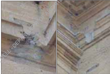
Figure 75 (a, b). Inappropriate Repairs of Damaged Cornices
