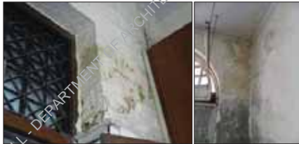
Figure 64 (a, b). Seepage and Paint Blistering of walls
