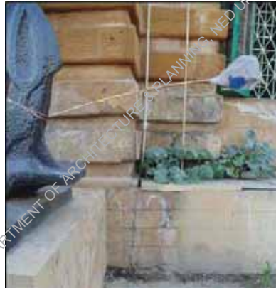
Figure 65. Macro biological Growth due to Faulty Plumbing Services
