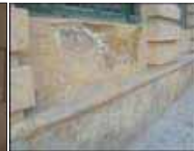
Figure 63. Disintegration and Exfoliation of Plaster and Stone Surface
