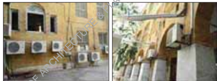
Figure 82 (a, b). Haphazardly placed AC units on building rare side
