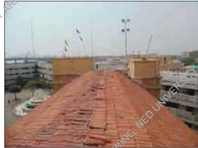
Figure 88. Broken Roof Tiles
