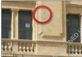
Figure 70. Iron Nails on Front Façade
