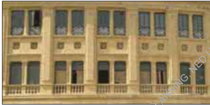
Figure 74. Affected Windows of Front Facade
