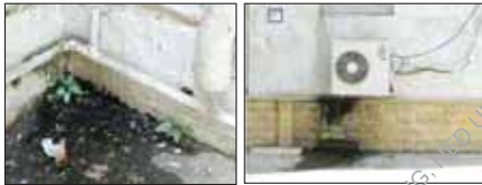
Figure 66 (a, b). Microbial growths due to dampness
