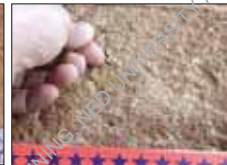
Figure 52. Crumbling of Stone
