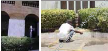
Figure 55(a, b). Hedges along building periphery, marble cladding & rising damp
