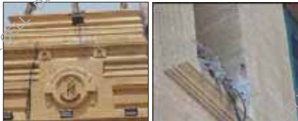
Figure 79(a, b). Birds Droppings and Bird's Nest in Window of Front Facade
