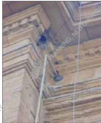
Figure 56. Inappropriate Plumbing Services on Front Façade
