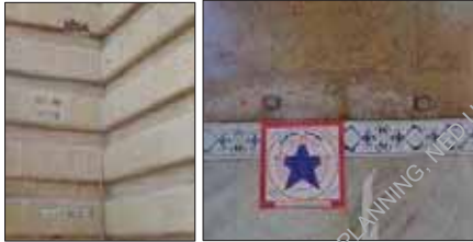
Figure 87 (a, b). Wooden Insertions in Slope
