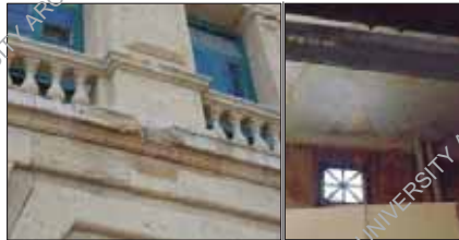
Figure 57 (a, b, c, d, e, f). Dampness due to faulty plumbing
