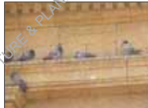
Figure 78. Birds Perching on Building Cornices
