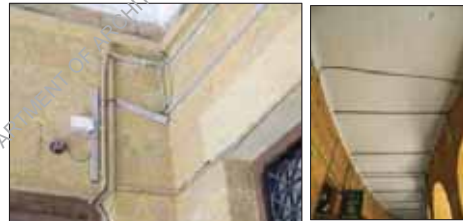
Figure 80 (a, b, c). Exposed Faulty Electric Wiring inside Corridor
