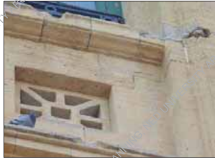
Figure 76. Inappropriate Repairs of Damaged Cornices
