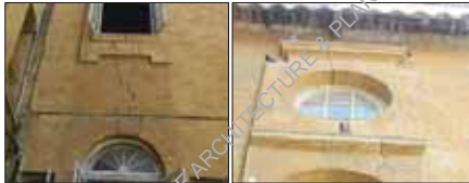
Figure 58 (a, b). Cracks in Stone Surfaces
