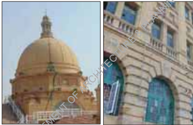
Figure 81 (a, b). Exposed Electric Wires on Dome & Front Facade
