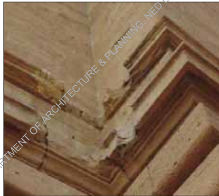
Figure 73 (a, b). Broken Cornices
