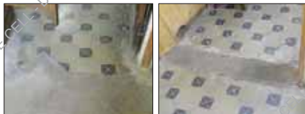
Figure 83 (a, b). Improper Floor Repair with Cement
