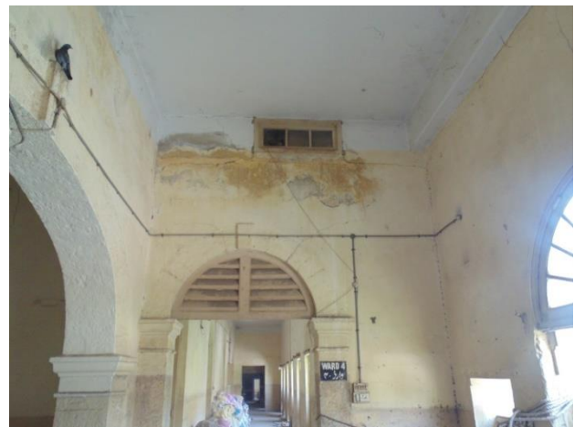
Figure-51 Cracks on the Walls of First Floor Corridor
