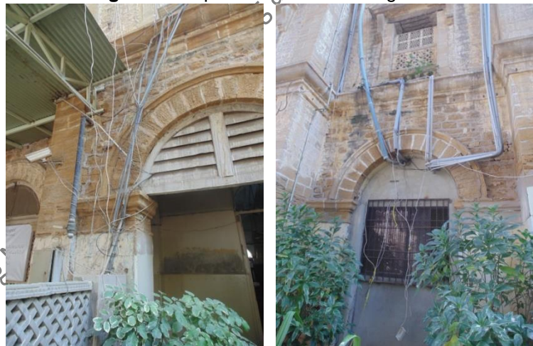
Figure-33 a, b Exposed Wiring on Façade
