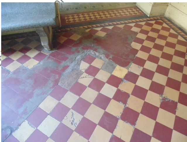
Figure-42 Inappropriately Altered Geometric Patterns
