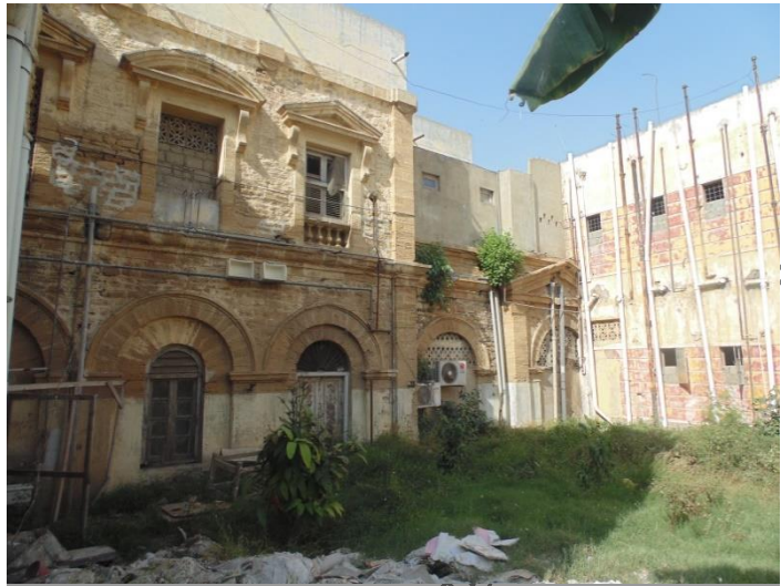
Figure-43 Exposed Plumbing, Water Pipes and AC Units
