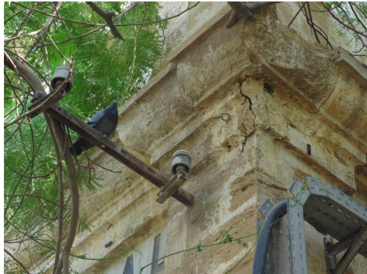
Figure-32 Exposed Electrical Wiring
