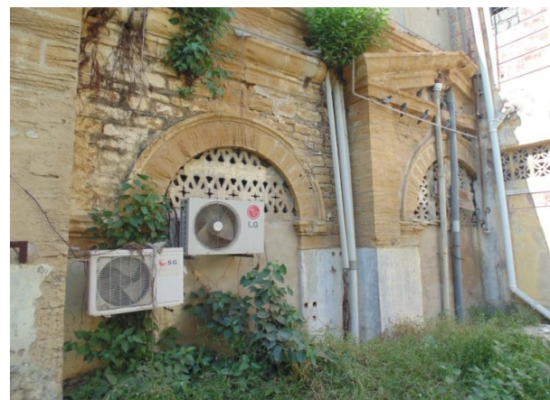
Figure-31 AC Unit Attached with Stone Wall
