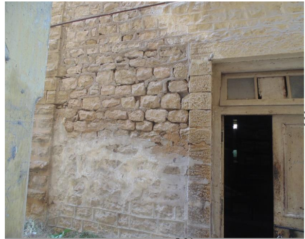
Figure-46 Open Mortar Joints on Record Room Block
