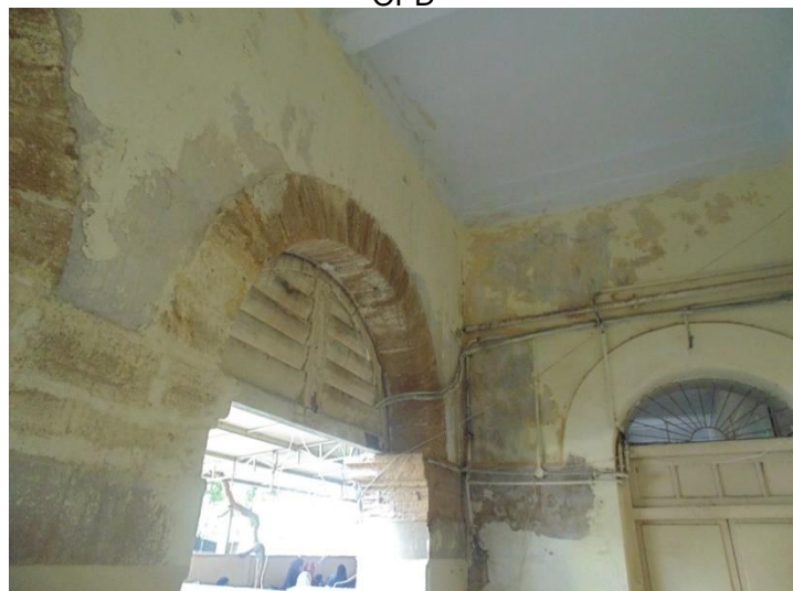
Figure-45 Moisture Stains Inside the Corridor
